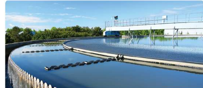
Water Treatment Plant - Tender has been awarded to SPML of INR. 90 Cr. A water treatment plant of 50 MLD will be established.
