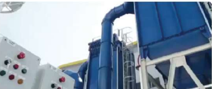
Common Effluent Treatment Plant (CETP) - A CETP is required in Dholera Industrial City - Tender has been floated for the same & bidding is under progress for a 20 MLD CETP.
