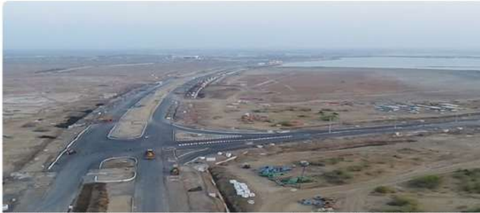
Roads and Services - Tender has been awarded to L&T of INR. 1734 Cr. L&T has mobilised on site & work has already commenced.
